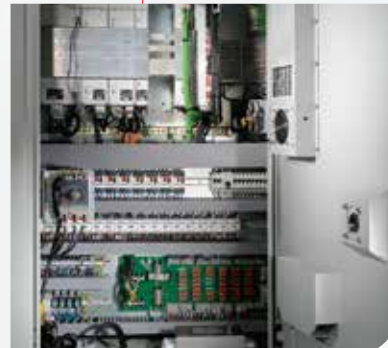
ELECTRICAL COMPONENTS ARRANGED IN MODULAR DESIGN FOR EASY MAINTENANCE
